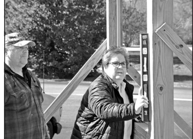
Mayor Ordiales with Dave Seddon a couple weeks back, during the construction of the sign.
