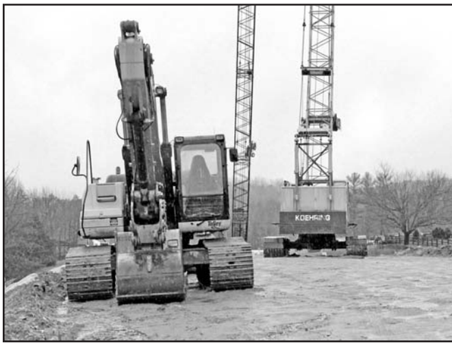
Photo by Shawn Jarrard Bridge replacement construction has already begun, and the new bridge will be higher and to the west of its former location.
