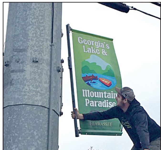
Heath Moss, with the Hiawassee Wastewater Treatment Plant, hangs one of the Hiawassee Business Group’s long-promised seasonal banners. Moss had help from Carl Grizzle, who drove the forklift that raised him during the installation.
