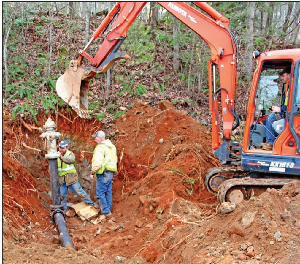
County workers are installing fire hydrants at a record pace. Only the weather is keeping these important infrastructure pieces from being installed any faster. Photo/Marty Roberts
