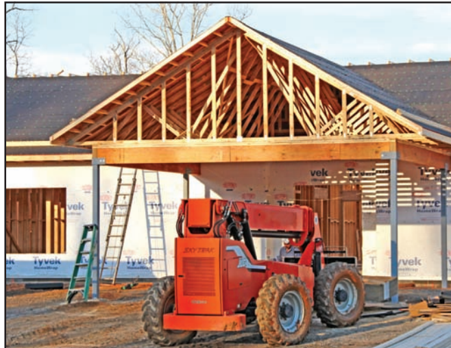
From pouring the foundation to drying in the building, the new Senior Center is on pace to meet the 180 days or so construction deal with the county. Photos/Marty Roberts
